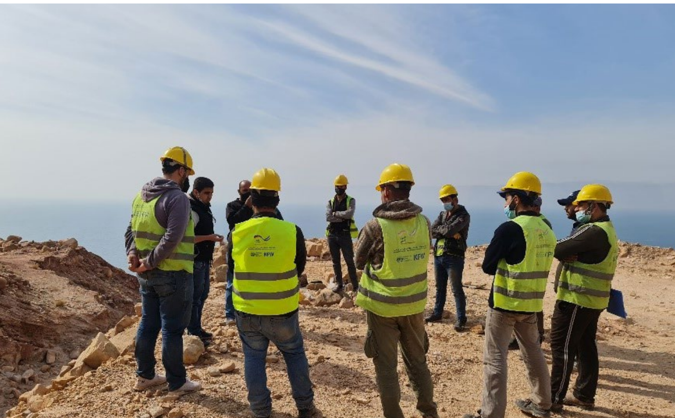
Workers on the KfW-funded Employment Intensive Investment project (EIIP) in Jordan receiving their site safety briefing and duties description from their supervisor on the eastern bank of the Dead Sea, in cooperation with the Ministry of Public Works and Housing
