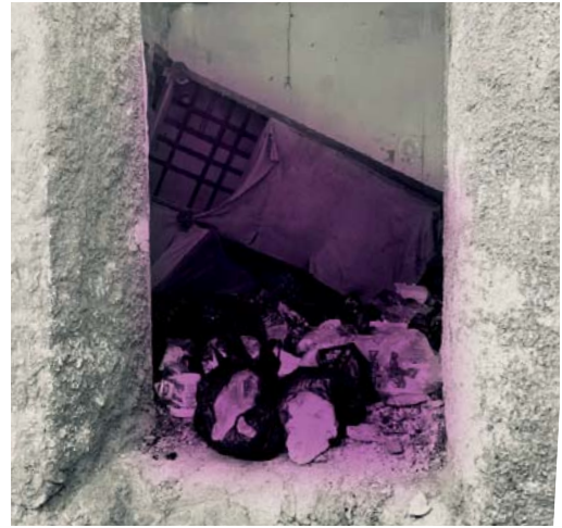
Health Hazardous Area
